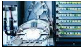
Optical Distribution Frames
