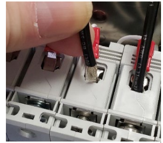
Figure 8 Connecting the load
