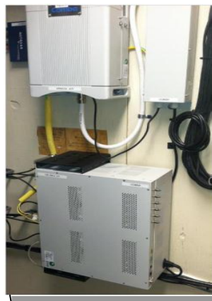
mBDA, ComFlex MU and RU Installation Main Equipment Room
