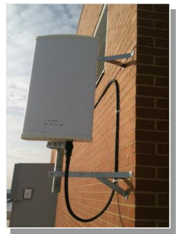
Single Port Donor Antenna Installed on Roof
