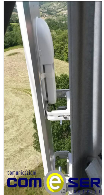
ePMP Access Point connects a community
